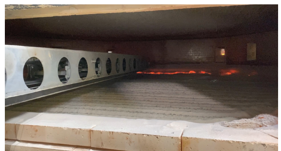
Figure 3: Cold top charger over batch blanket in a cold top vertical melter.
